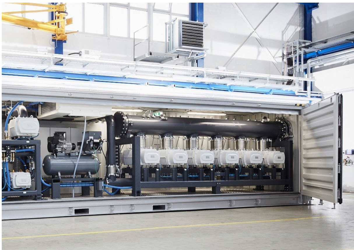
Figure 1: Container-based vacuum pump system as delivered by Leybold.
